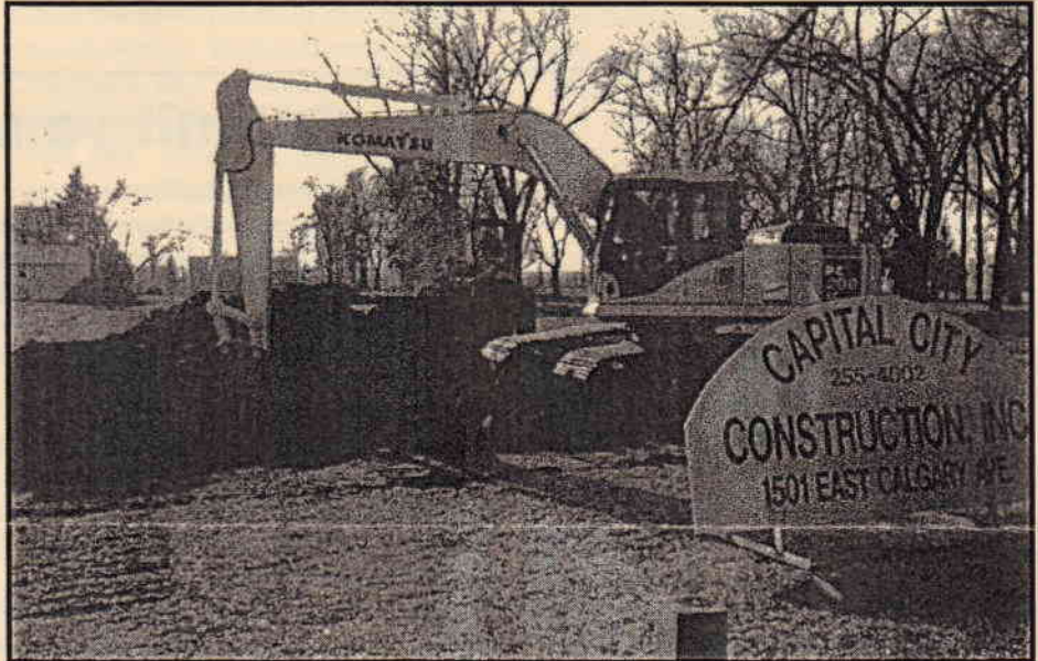
Excavation work began on a new UTTC dormitory following groundbreaking on December 9. The building will house 86 students and is located near the cafeteria, just west and slightly south of the campus security building.
