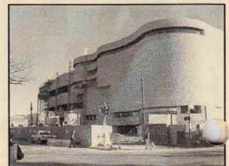
Under construction in the nation's capitol is the National Museum of the American Indian, set to open September 21, 2004.
