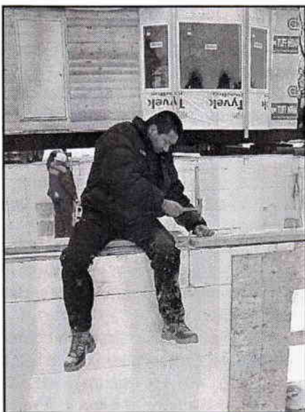
Carpentry student Richard Scott, Fort Mojave, CA, sits atop the foundation wall to chisel room for anchor bolts in the sill plate before the building is moved into position.
