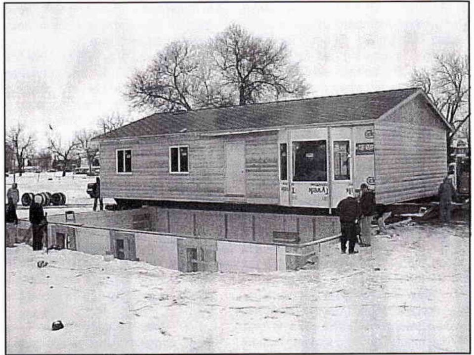
Below zero wind chill temperatures on January 23 tested UTTC students and workers from House Movers of Minot, ND when moving the 1,248 square foot building from the Skill Center onto its foundation on the north side of campus.
