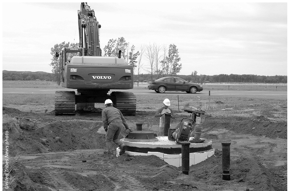
Construction work began in April along University Drive on the infrastructure for the new campus at United Tribes Technical College. A dedication ceremony is scheduled for September 5.
