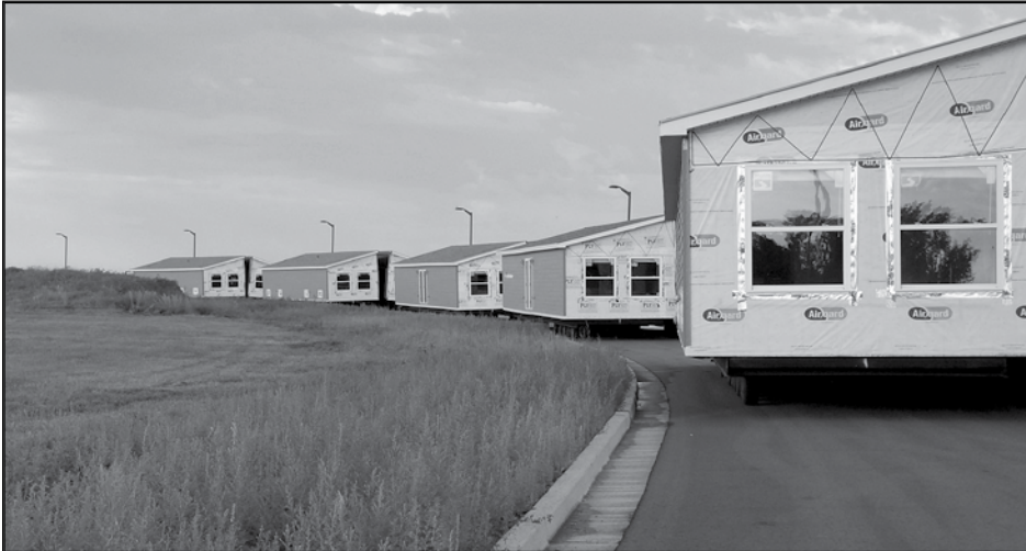
ALL IN A ROW: A group of modular classroom units are staged and ready to serve in the expansion of Theodore Jamerson Elementary School on the United Tribes campus. The units were parked in July on a roadway of the college's new south campus, awaiting site preparations at an area along Sisseton Street on the east side of the original campus. TJES serves the children of college students who attend United Tribes. United Tribes News photo Dennis J. Neumann
