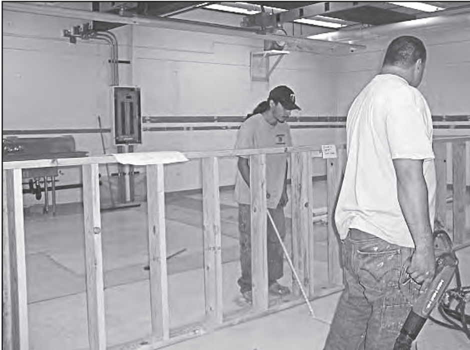
UTTC construction students Steve Raining Bird and Cameron Johnson are building a new dividing wall in the "gutted" Nutrition and Foodservice Kitchen.
