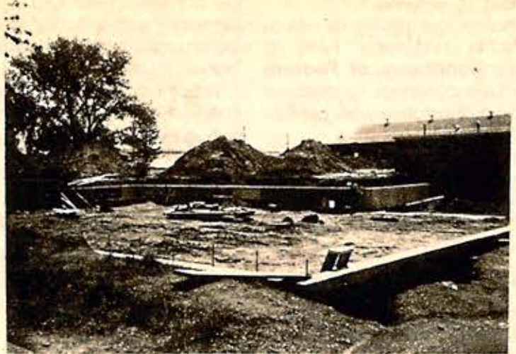
Another photo of the gymnasium area. This section of the building will contain a regulation size basketball court and will also be wide enough to play 2 cross count basketball games and/or volleyball.
