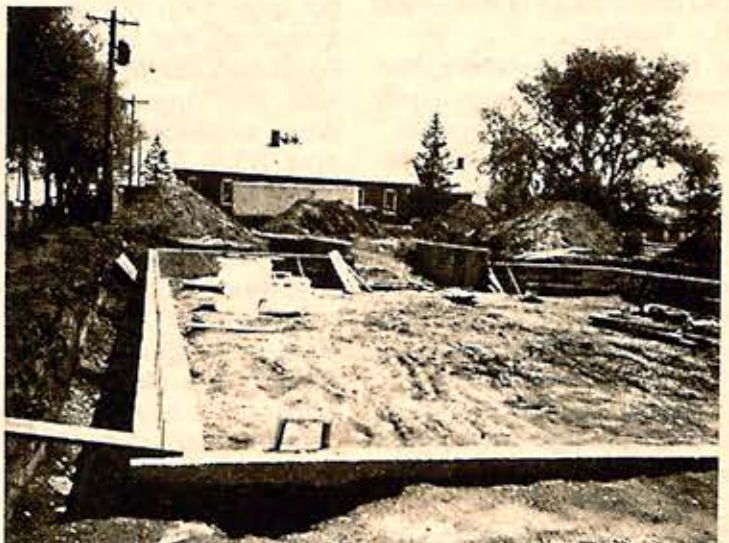
The above picture shows the area where the gymnasium floor will be. At the back of the building will be a garage door, making it possible to move equipment in and out.
