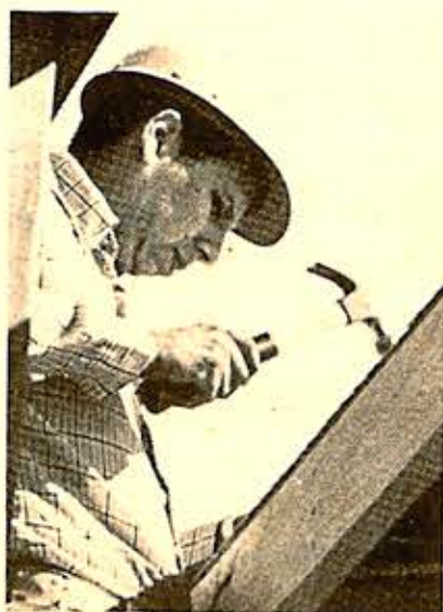
Norman Stewart, building trades student, nails down the roofing after Charlie Huber [driving fork-lift] helps other UTETC students put the plywood sheets in place.
