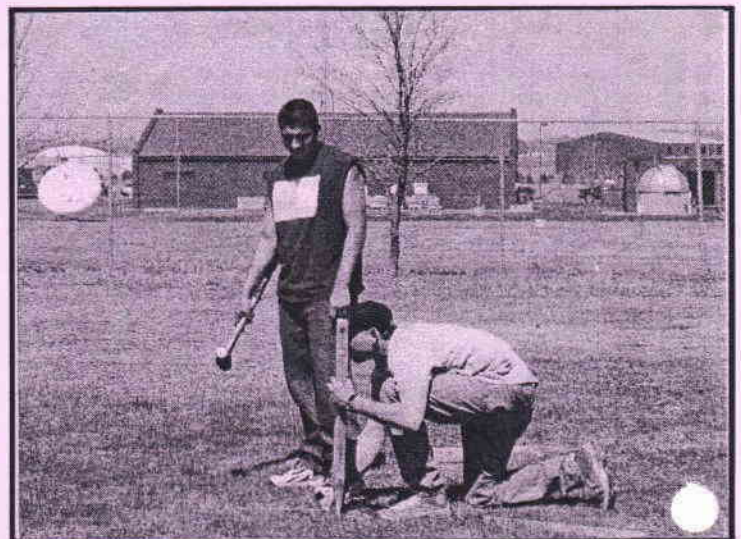
Construction Technology students Anthony Quick Bear and Deeken Means siting and staking the area for the new UTTC Log Cabin Interpretive Cultural Arts Center.
